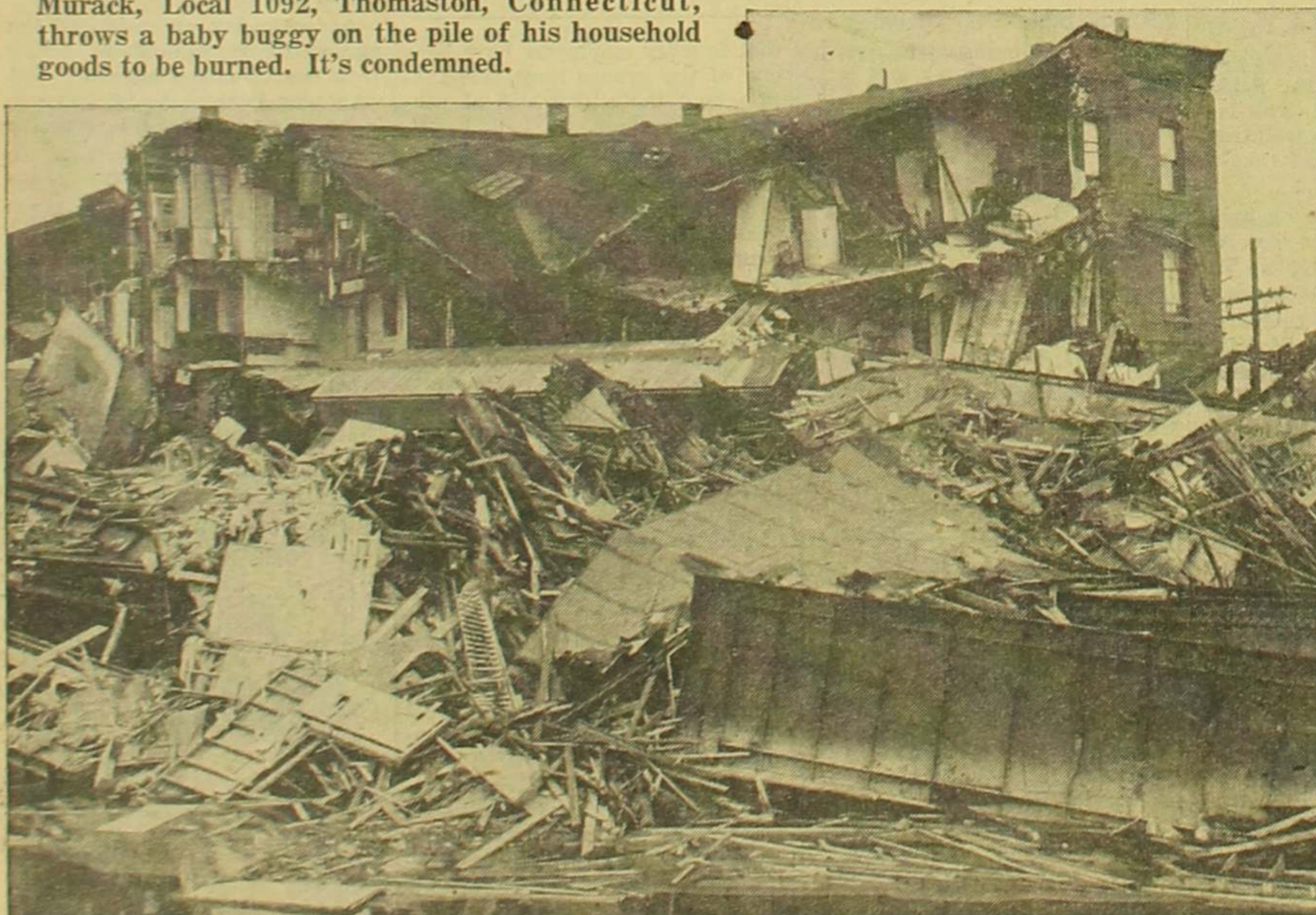
THIS IS WHAT RAGING WATER can do to a brick apartment building. A boxcar, swept along by the torrent crashed into the side of this structure, which housed some UAW families in Torrington, Connecticut. It caved in immediately. Notice the refrigerator which miraculously stays in place in the upper right apartment. Some homes were lifted from their foundations and sent swirling down the Naugatuck Valley. Nearly every community in the Valley suffered damage like this.
