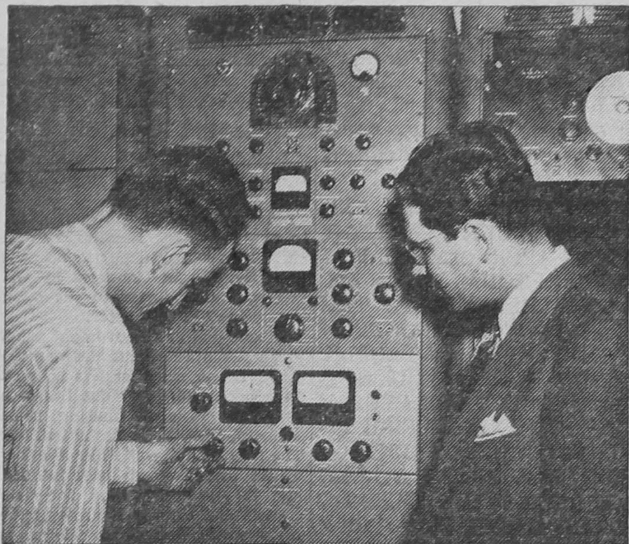
Chief Engineer Lester West, left, and Station Manager Ben Hoberman, check newly-installed equipment at Radio Station WDET.
